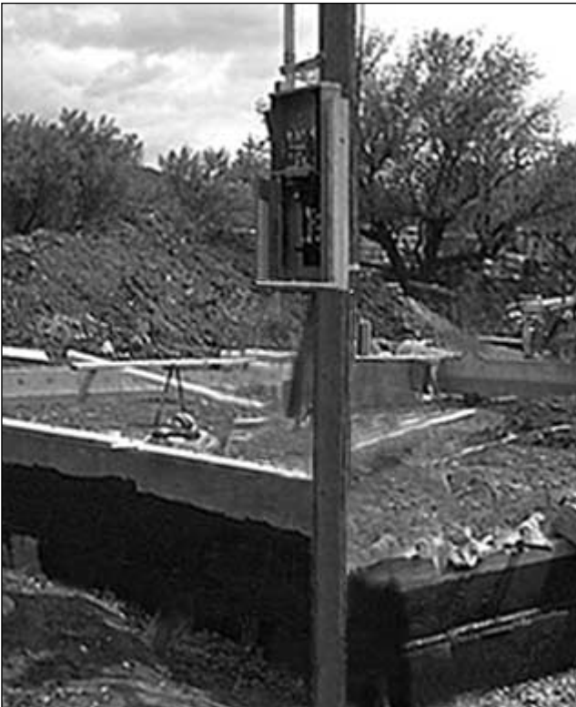
FIGURE 2.1 Example of temporary power for new construction.
