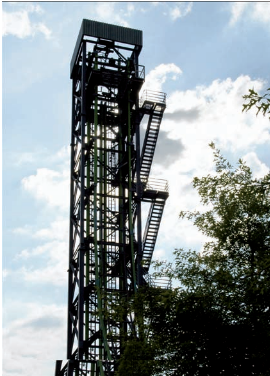
Figure 10-8: The corrected tower looks like this.
