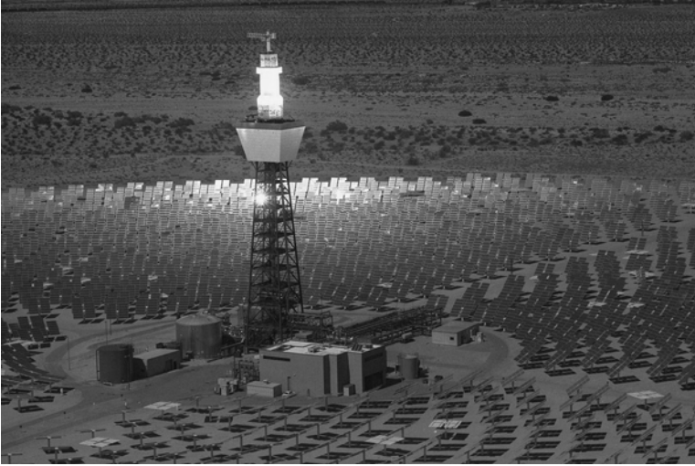
Figure 7.1 “Solar Two” concentrating solar power plant. Source: DOE.
