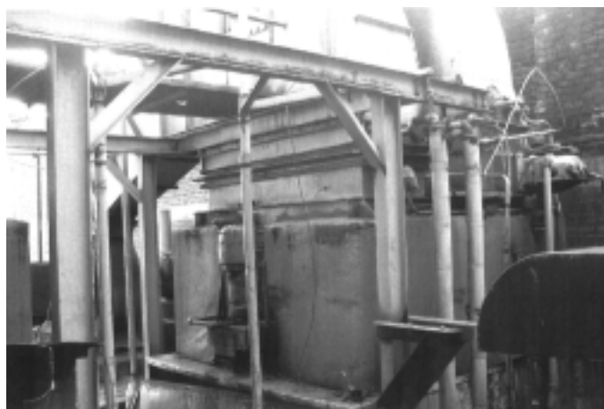
Figure 9-42. Lungstrom air preheater
