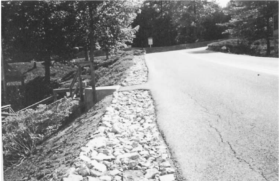
Figure 6.8 Photograph of a swale infiltrator.
