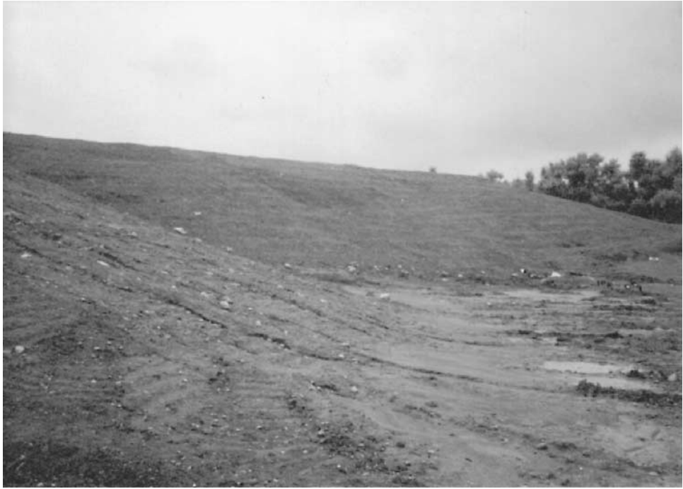
Figure 7.2 Photograph of tracking on a slope.
