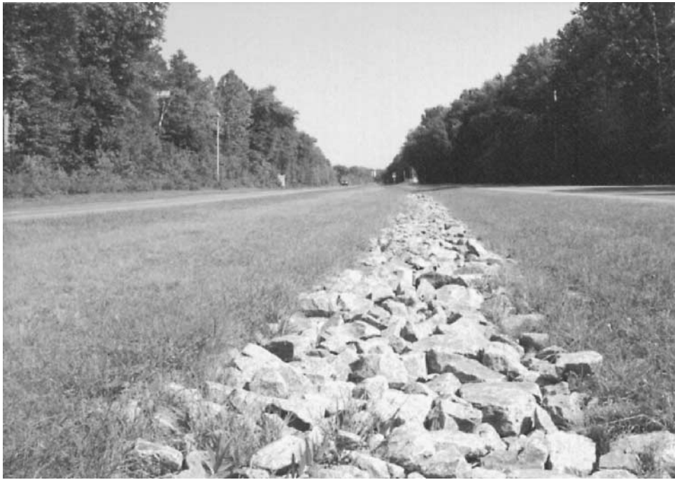
Figure 6.16 Photograph of infiltration trench in median.
