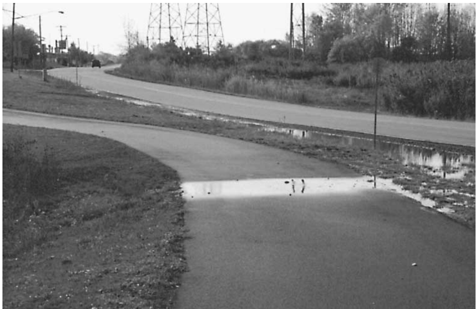
Figure 4.46 Photograph of path surface with pooled or standing water.
