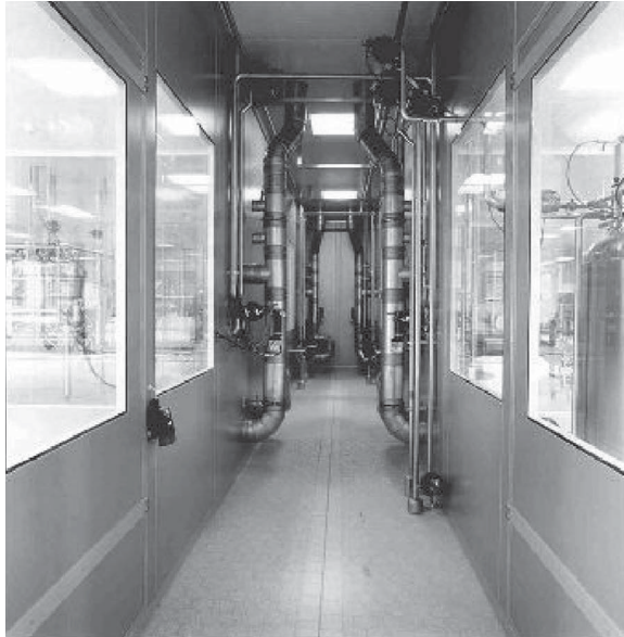
FIGURE 19 The utility chase is located between two clean rooms. Major utility lines are installed within the chase and hook-up lines for local pieces of process equipment are connected through the clean-room walls. A major benefit of this arrangement is that installers need not be fully garbed in clean-room attire to access the utility lines. (Courtesy of CleanTek.)
