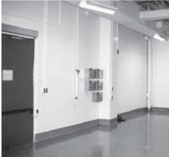
FIGURE 6 A CMU wall treated with block filler and epoxy finish to provide a smooth, cleanable wall surface. (Courtesy of Niagara Walls.)
