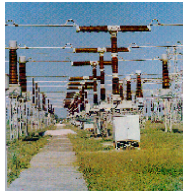
Live bank breaker (Courtesy BHEL)
