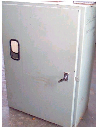
Fig. 17.3: Mechanism box with local control unit
