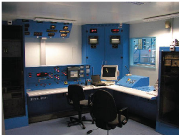
Figure 25 MINERVE reactor control room
