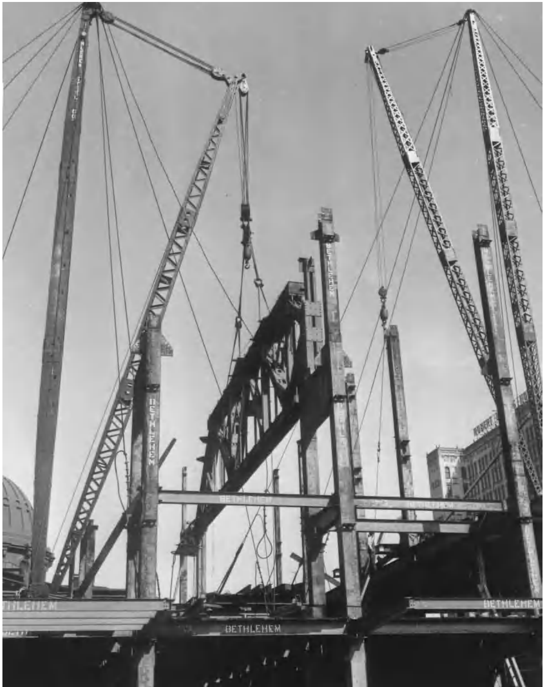
Fig. 1. Steel erection with guy derricks on a high structure. (Bethlehem Steel Co.)
