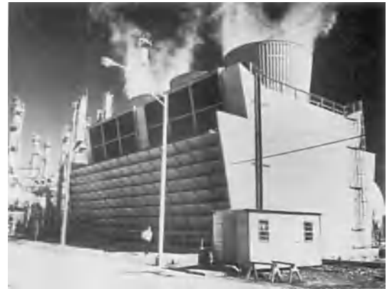
Fig. 5. Wet-dry cooling tower at Atlantic Richfield Company. (Marley Co.)
