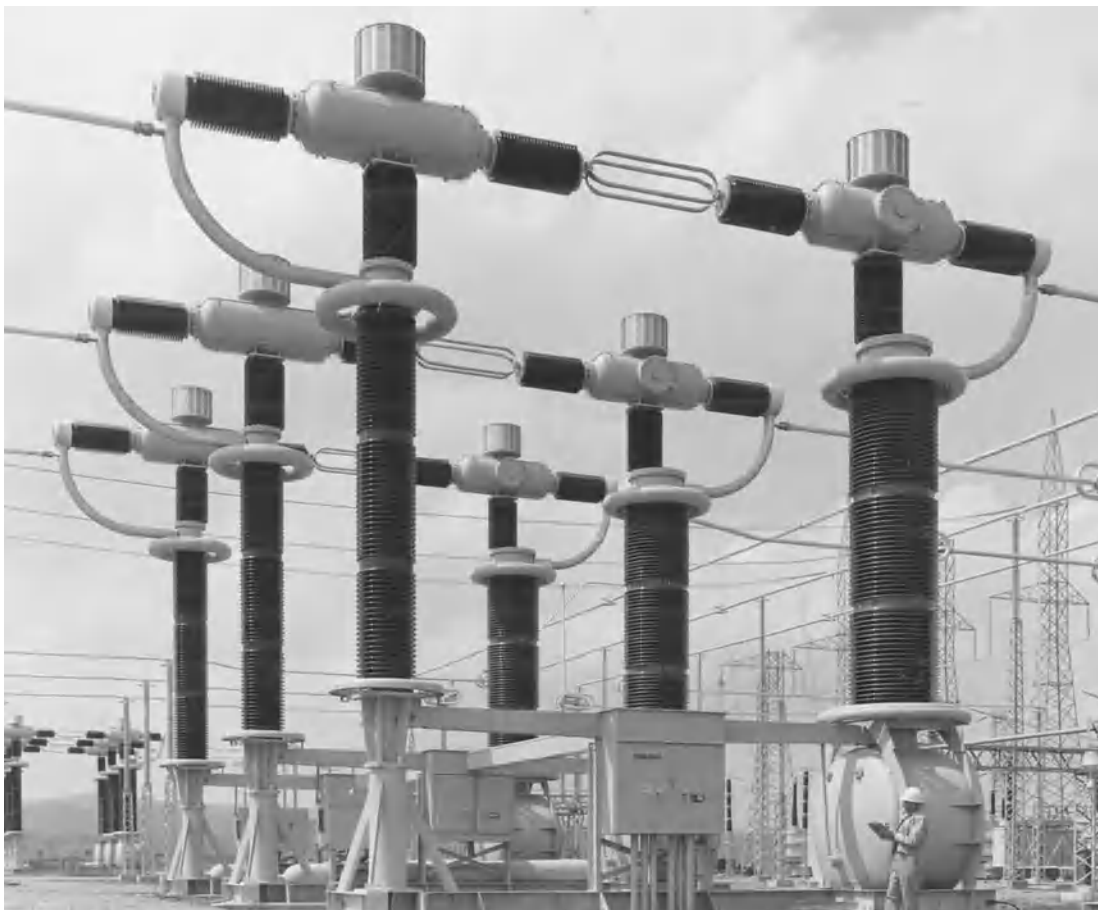
Fig. 3. Air blast circuit breaker rated for 500 kV.
