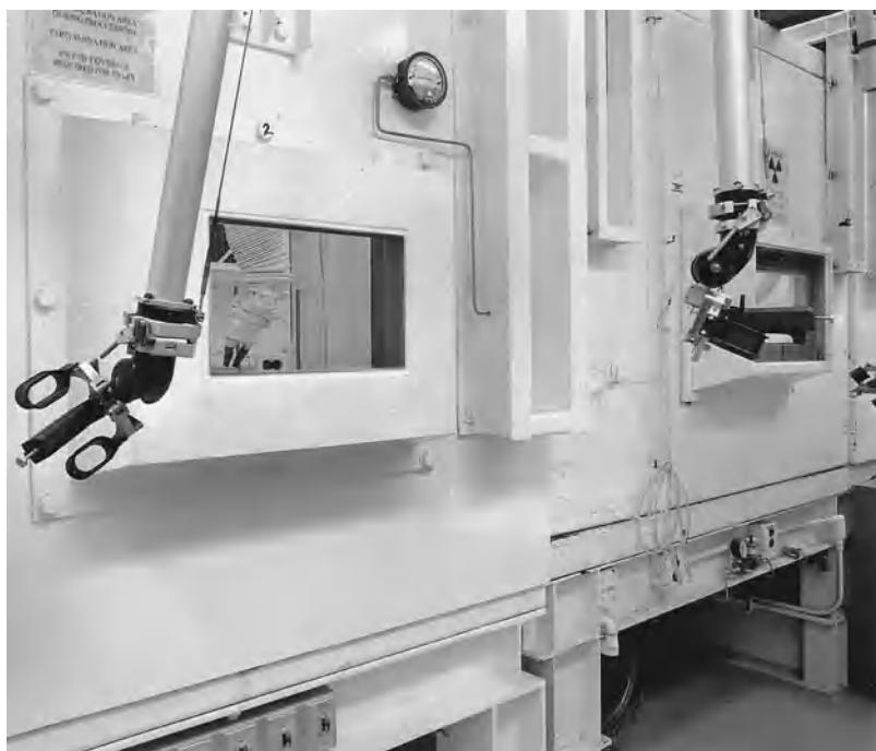
Fig. 3. Exterior view of two hot cells with manipulators. The walls are 7-in.-thick (17.75-cm) lead, encased in 1/4-in.-thick (0.6-cm) steel plate. The lead glass windows are 14 in. (35.5 cm) thick and provide shielding equivalent to the walls. (Brookhaven National Laboratory)
