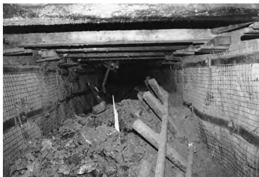
Rock burst damage to a mine opening from a small pillar burst. Note the track and rail heaved up almost 8 ft (2.5 m).
