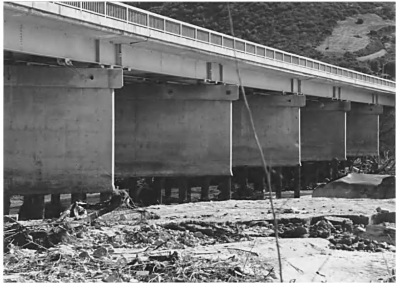
Fig. 3. River bed scour at a bridge crossing induced by sand mining in the river channel.
