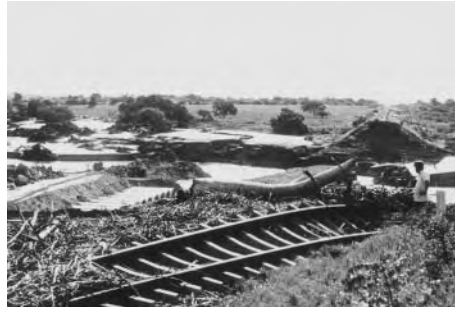
Plate 5 The demolition of a railway line in Swaziland, southern Africa, caused by floods associated with a large tropical cyclone. One role of the applied geomorphologist is to undertake post-event surveys in order to ascertain past discharges
