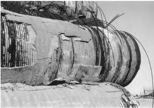
Plate 106 Damaged water pipelines in central Namibia. They proved to be unable to withstand the corrosive conditions associated with the foggy, salty environment of the Namib, and had to be replaced after only a few years in service
