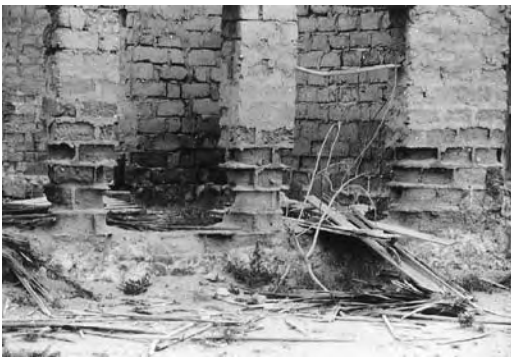
Plate 108 Concrete buildings in Ras Al Khaimah, United Arab Emirates, illustrating salt weathering caused by migration of salt solutions up the pillars by the wick effect. The process is exacerbated by high ground water levels associated with the spread of irrigation
