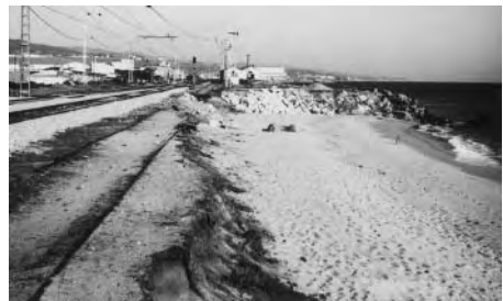
Plate 55 The main railway line between France and Spain near Barcelona. Note the severe erosion of the coastline, and the abandoned track in the foreground. Sandy beaches of this type will be especially sensitive to the effects of accelerated sea-level rise associated with global warming
