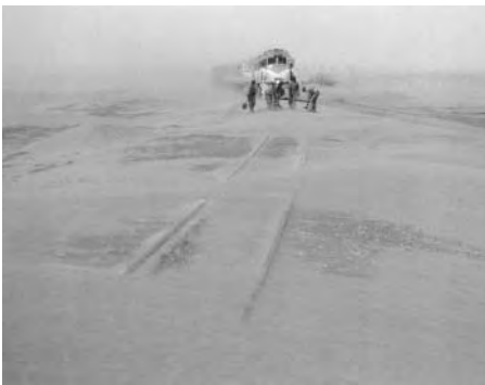
Plate 4 The main railway line from Swakopmund to Walvis Bay in Namibia illustrates the hazard posed by sand and dune movement. One role of the applied geomorphologist is to identify optimum route corridors and to advise on their management
