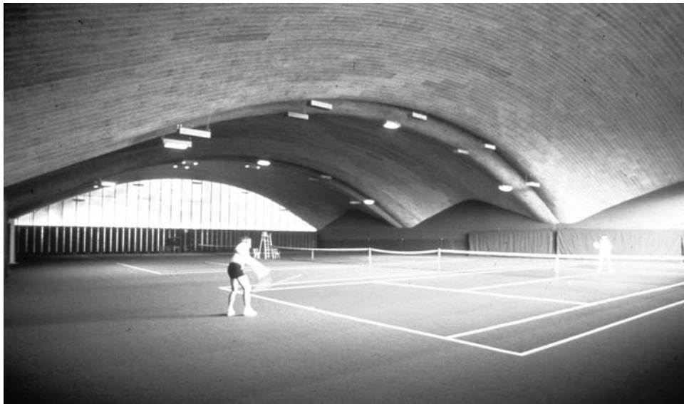
Figures 20 & 21. Reusable formwork for a shell roof over an indoor tennis court, near Norwich, England by Heinz Isler. [Photos: Heinz Isler, Tony Copeland.]
