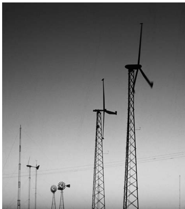
Figure 4. At the USDA-ARS Conservation and Production Research Laboratory in Bushland, Texas, wind turbines generate power for submersible electric water pumps that are far more efficient than traditional windmills (background).
