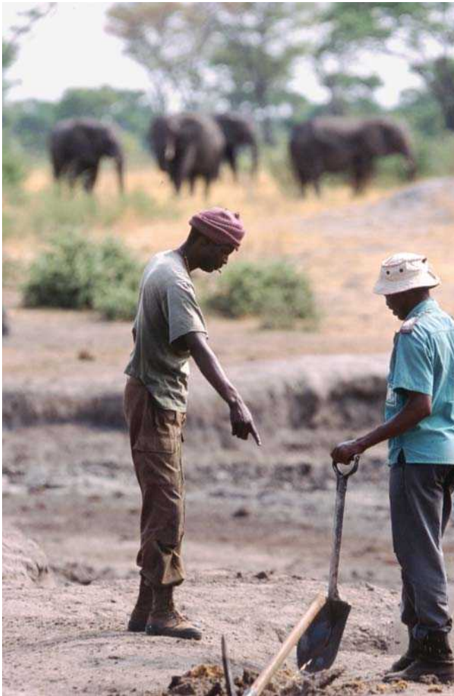
Wardens fix water pipes in Khaudum Game Reserve, in Namibia, as elephants in the background wait for water. (Photo by Rudi van Aarde. Reproduced by permission.)
