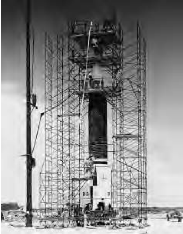
This historic photograph shows the construction scaffolding used to create a contemporary gantry at Cape Canaveral Air Force Station in July 1950 to help workers prepare the Bumper 8 rocket for launch. (Bumper 8, the first rocket shot from Cape Canaveral, was a captured German V-2 rocket modified by American rocket engineers.) (Courtesy of the U.S. Air Force)
