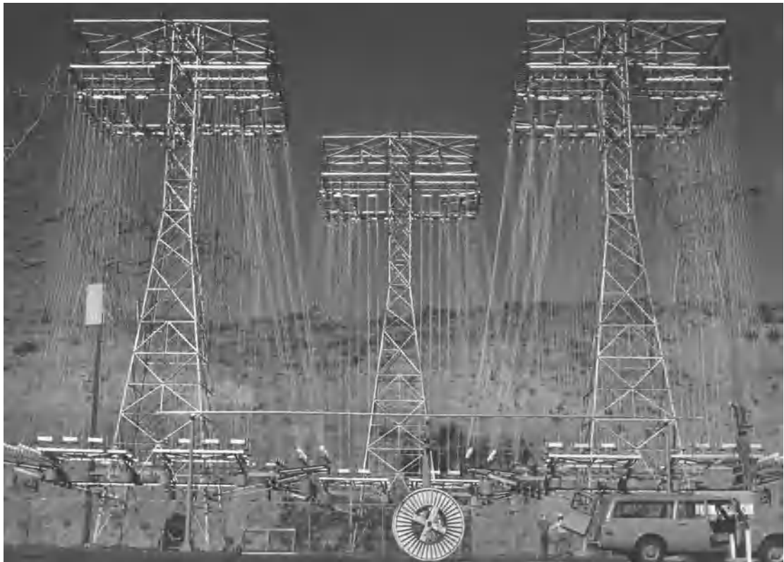
Dynamic braking resistor with a capacity of 1400 MW, installed in the Bonneville Power Administration's Chief Joseph Substation. (From M. L. Shelton et al., Bonneville Power Administration 1400-MW braking resistor , IEEE Trans. Power Apparatus Sys. , PAS-94:602-611, Institute of Electrical and Electronics Engineers, 1975)
