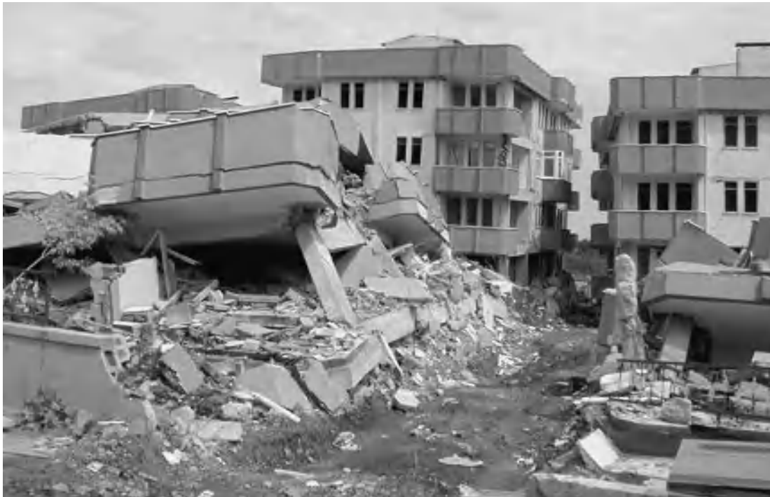
Fig. 1. Relatively new reinforced concrete buildings that collapsed in the Marmara, Turkey, earthquake, August 17, 1999.
