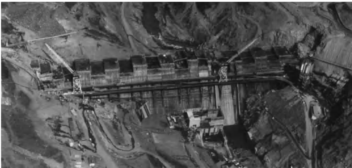
Fig. 9. Block method of construction on a typical concrete gravity dam. (U.S. Army Corps of Engineers)
