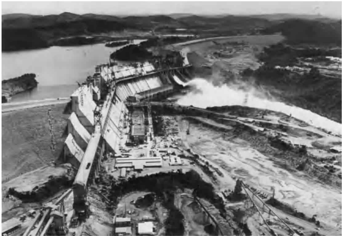
Fig. 3. Guri Dam, Venezuela, showing construction under way on the second stage of the concrete gravity dam. Embankment dams are shown on the left and right abutments. The concrete batch plant is shown at left with a trestle for transporting concrete shown on the downstream face of the dam. The second powerhouse with an excavated outlet channel is shown at the center of the photo. (C.V.G. Electrificación del Caroni, C. A. EDELCA, Caracas, Venezuela)
