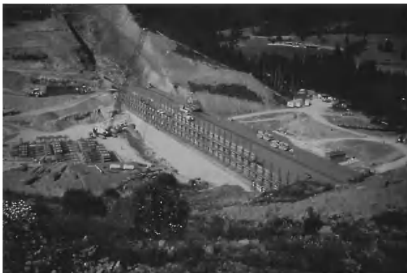
Fig. 13. Galesville Dam, Oregon, showing roller-compacted concrete construction; completed in 1985, it has a height of 157 ft (48 m) and a volume of 161,000 yd 3 (123,100 m 3 ).
