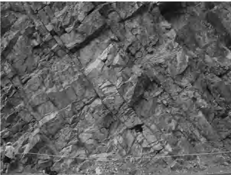
Fig. 1. Typical rock mass containing numerous discontinuities. The person in picture is conducting a scanline survey, where a tape is placed across the rock and detailed information is gathered on the fractures that intersect the scanline.
