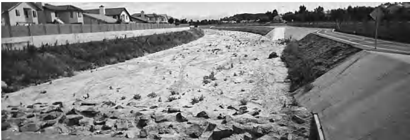
Fig. 2. Channelization of the Santa Gertrudis Creek in California showing bank protection and grade control structure traversing the channel bed.
