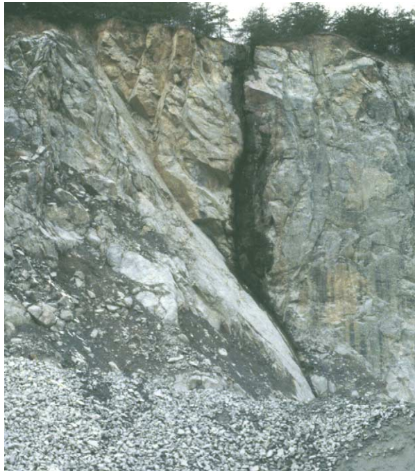
Figure 1 Quarry operated for construction aggregate, road metal, and granular fill, in dolerite (diabase) and high-grade crystalline metamorphic country rock of Prince George's County, Maryland, USA; the vertical face is approximately 15 m high. The pit has reached the lateral limits of the deposit of usable rock and also has come to the maximum viable depth for maintenance of the pit, removal of groundwater seepage, and precipitation runoff. The site was being considered for conversion to a long-term secondary use compatible with environmental protection requirements. Photograph by the author.
