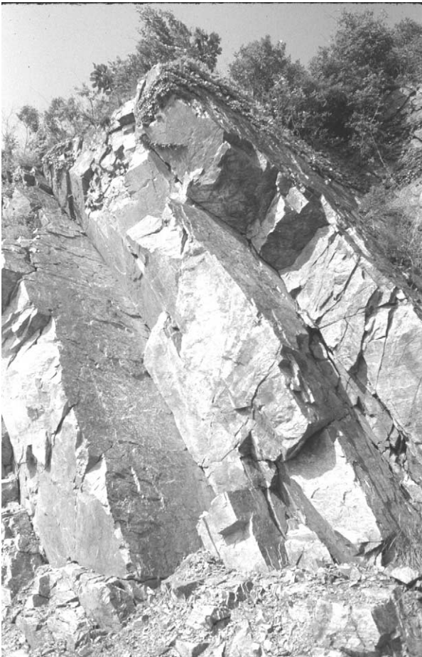
Figure 2 Rock highwall in rhyolite near Munsan, Republic of Korea, exhibiting three prominent joint sets of consequence to development of the site as a quarry. Such features should be taken into direct consideration in quarry dimensioning and in specification of the bearings of bounding highwalls; the horizontal width of the exposed joint faces is about 5 m, left to right. Photograph by the author.
