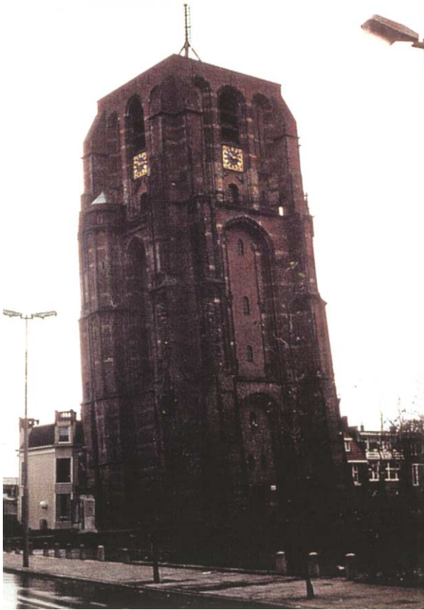
Figure 3 Leaning church tower due to differential settlement in soft Holocene sediments, a foundation problem near Lake IJssel, The Netherlands. de Mulder EFJ, Holland, International Union of Geological Sciences 'COGEOENVIRONMENT' photograph.
