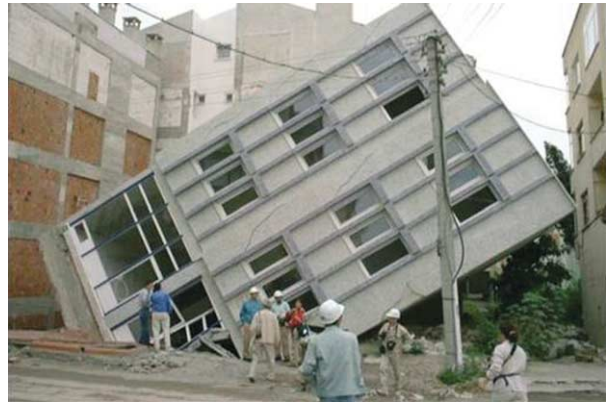
Figure 13 Tilted apartment block in Adapazari, Turkey, due to extensive liquefaction in the 1999 magnitude 7.4 Kocaeli earthquake. This building had thick, continuous, shallow foundations, which caused it to rotate as a rigid body. There is very little damage to load-bearing elements, walls, or ceilings; nonetheless, the building would have been demolished. Photograph by Beyza Taskin.
