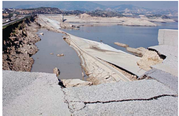
Figure 9 The failure of the upstream slope of the Lower San Fernando Dam shortly after the 1971 San Fernando earthquake. California narrowly avoided catastrophic flooding of 80 000 downstream homes. Liquefaction of the hydraulic fill caused loss of strength and slope instability, which left less than 1 m of freeboard after the earthquake. This picture shows the slide after emptying the reservoir; the paved road to the left indicates the former dam crest. Photograph by Leslie F. Harder, Jr.
