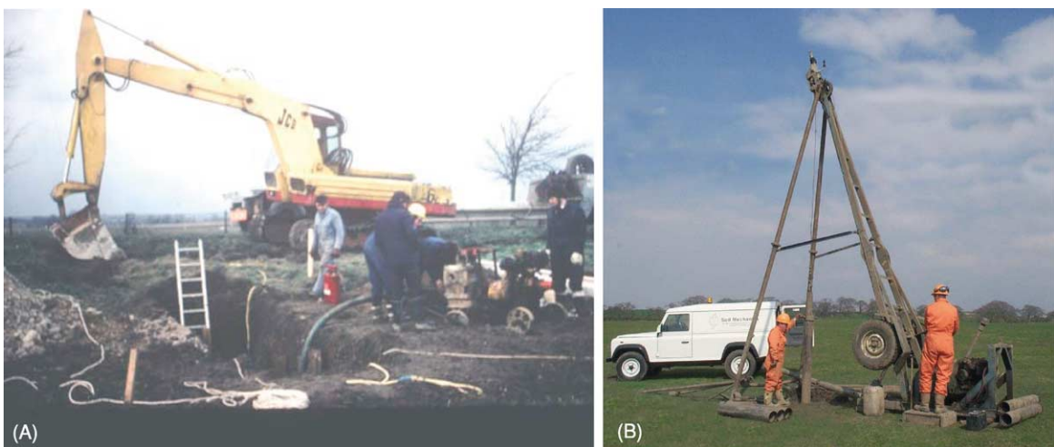
Figure 2 Two common methods of exploration. (A) The trial pit, with shoring and ladder for safe access and egress. (B) The percussion boring rig.
