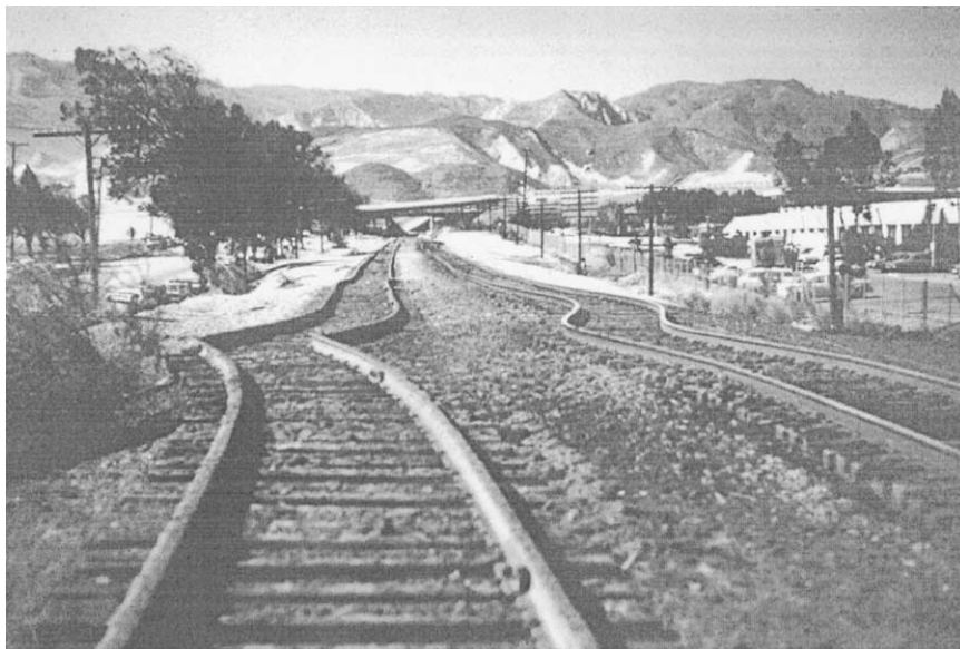
Figure 1 Engineering geological mapping records evidence of earthquake motion such as this railroad deformation indicating north-to-south shortening of the ground along the rail right of way. Most evidence of earthquake damage is fragile and likely to be destroyed by human activity within hours or days. (Photographed by Richard J. Proctor, then Chief Engineering Geologist, Metropolitan Water District of Southern California, at San Fernando Valley, California, February 1971.)
