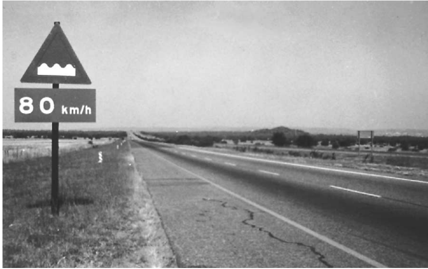
Figure 4 Breakup along the CapeTown Johannesburg road, South Africa, due to expansive clay.
