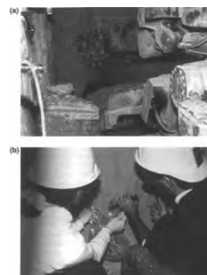
Figure 1. The Alpine miner was used to create passageways within the subsurface of Rainier Mesa, Nevada Test Site (a). The carbide bits on the rotating heads allowed rapid removal of relatively large volumes of rock without the necessity of drilling fluids or the production of excessive heat (b). After removal of large portions of rock, the Alpine miner was backed out of the alcove, and hand sampling was conducted with sterile implements (c).
