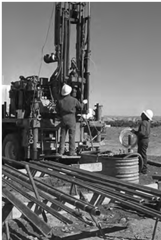
Figure 1. A typical truck mounted, rotary wireline coring rig operating at the Shiprock, NM uranium mill tailings site. At the time of the photograph, the rig was being used for installation and operation of straddle packers for conducting stress tests, for estimating in situ permeability of Mancos Shale, underlying the permeable terrace gravels. Samples for microbiology were obtained from both alluvial gravel deposits and Mancos Shale. See color insert.
