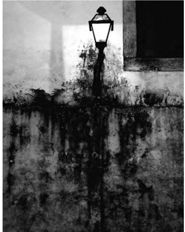
Figure 6. Intense algal growth behind a lamp attached to a building in Sao Joao del Rei, Brazil. Note black growth of mitosporic fungi in the rain runoff area below the lamp. See color insert.
