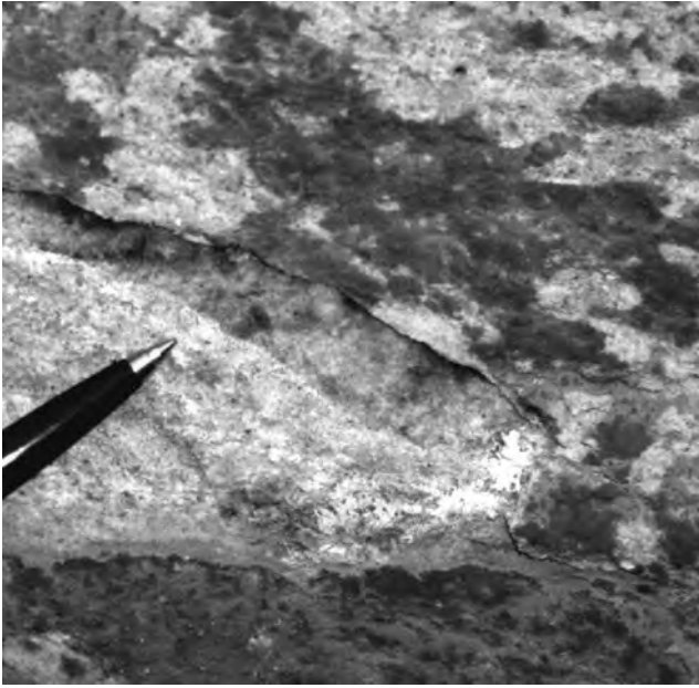
Figure 4. Spalled soapstone on the external wall of a church in Ouro Preto, Brazil. Cyanobacteria and actinomycetes were the major microorganisms detected below the detached layer. See color insert.
