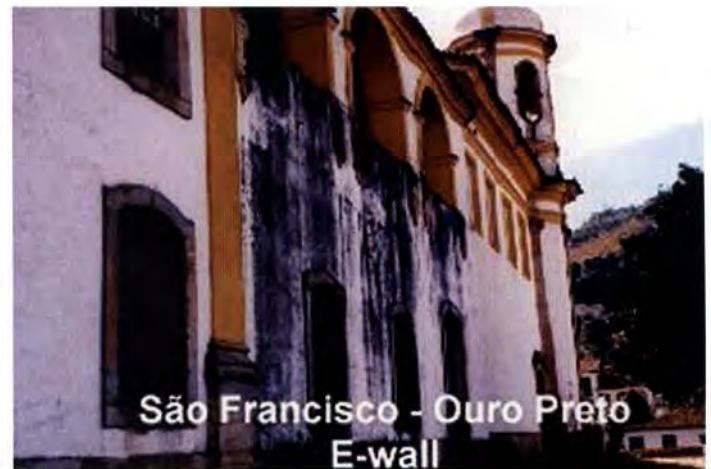
Biodeterioration of Mineral Materials, Figure 8. Intense black discoloration caused by growth of mainly mitosporic fungi and cyanobacteria on the east-facing painted wall of a church in Ouro Preto, Brazil.
