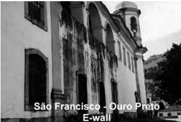
Figure 8. Intense black discoloration caused by growth of mainly mitosporic fungi and cyanobacteria on the east-facing painted wall of a church in Ouro Preto, Brazil. See color insert.
