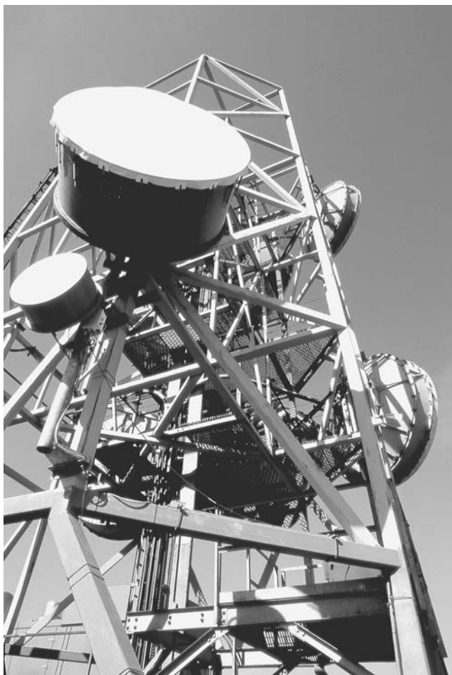
Satellite and cell phone towers have become ubiquitous in our age of communications.
