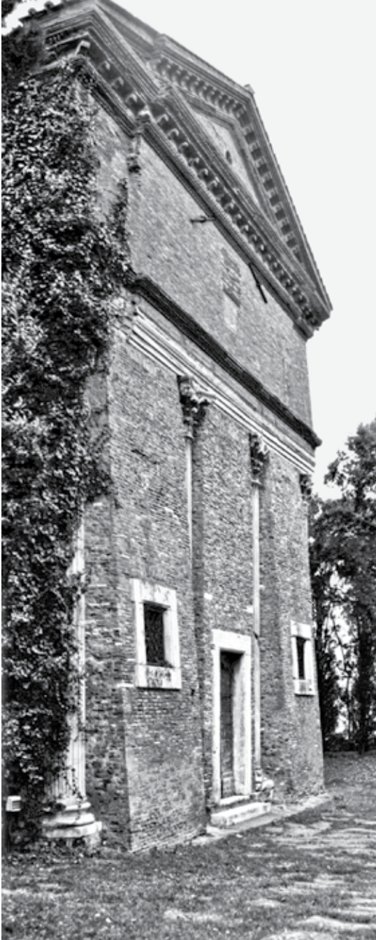
Figure 9.7. The exterior of S. Urbano, taken from the southeast; note the massive crack running from frieze to roof, no doubt necessitating the brink infill. Photo by the author, 1993.
