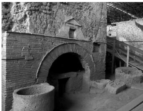
63. The large bread oven from the Bakery of the Chaste Lovers. Somewhat dilapidated, it still shows the cracks caused by the earthquake of 62 and the tremors that no doubt preceded the eruption.
